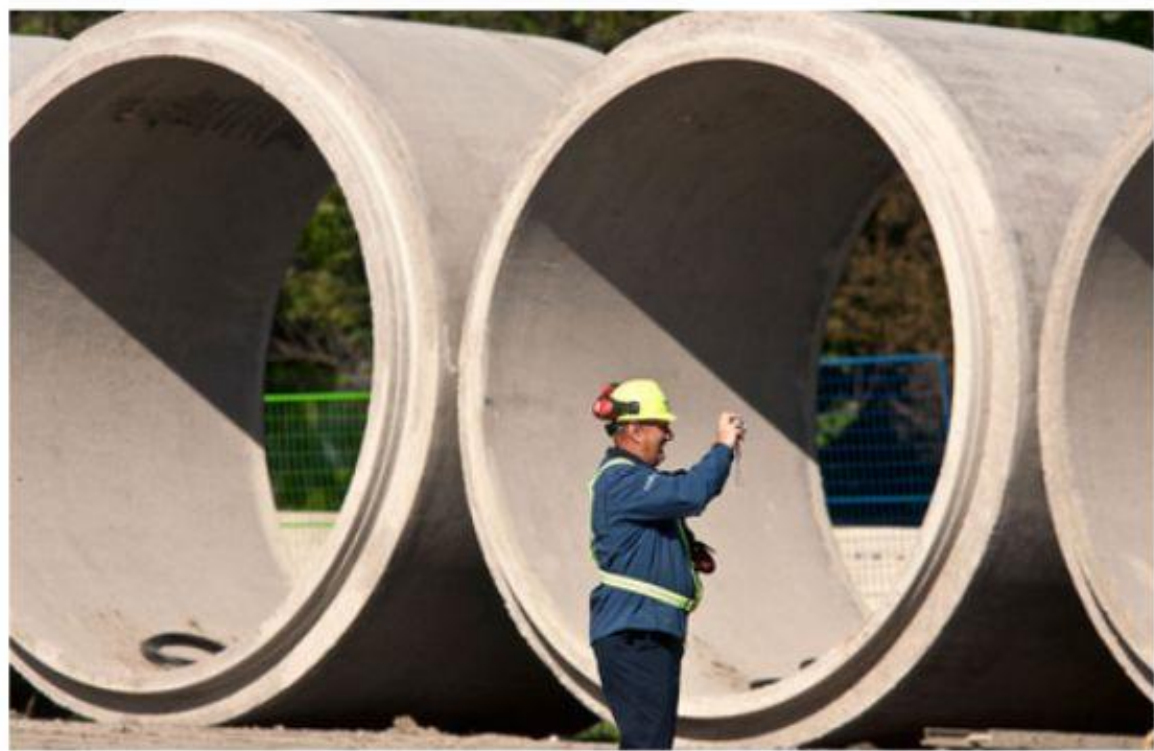
Work crews begin the installation of replacement pipe sections under the eastbound Highway 174 near the Jeanne d'Arc exit. This was the site of last week's sinkhole which swallowed a commuter's car.
